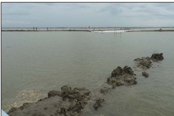
B. The high tide in the second week of June was too much for the temporary embankment and repairs.
