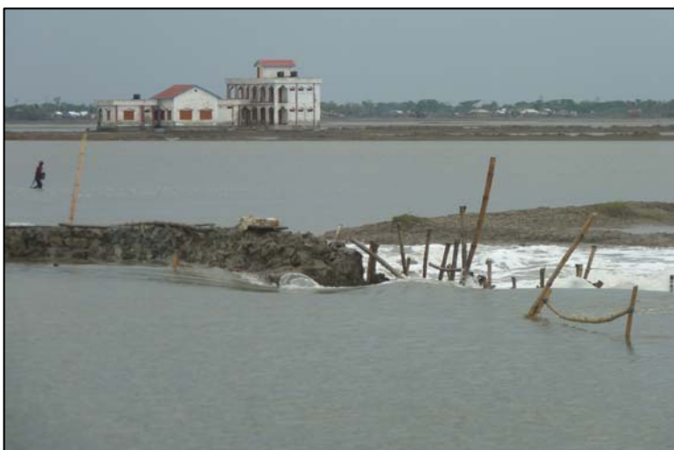
A. Saline water rushes into the Union following a breach of the temporary ring embankment which had been constructed after Aila had devastated the Union
